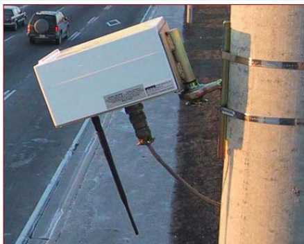
RTMS (Remote Traffic Microwave Sensor) radar
